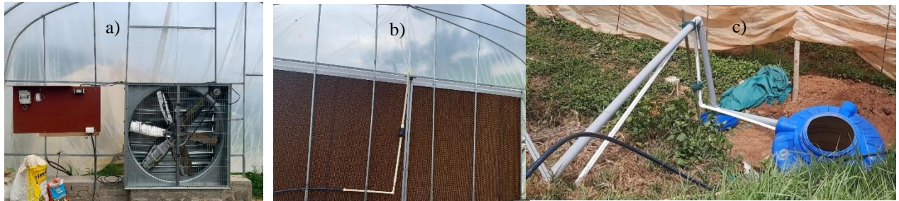
Figure 4. a) Installed exhaust fan and electrical point inside greenhouse b) cooling pad c) tank containing 500 litres of water connected to cooling pad through pipes.
