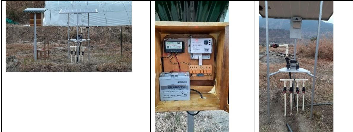
Figure 6. Installation of 2 HP pump and 100 watts solar panel for distribution of water into smart irrigation system.
